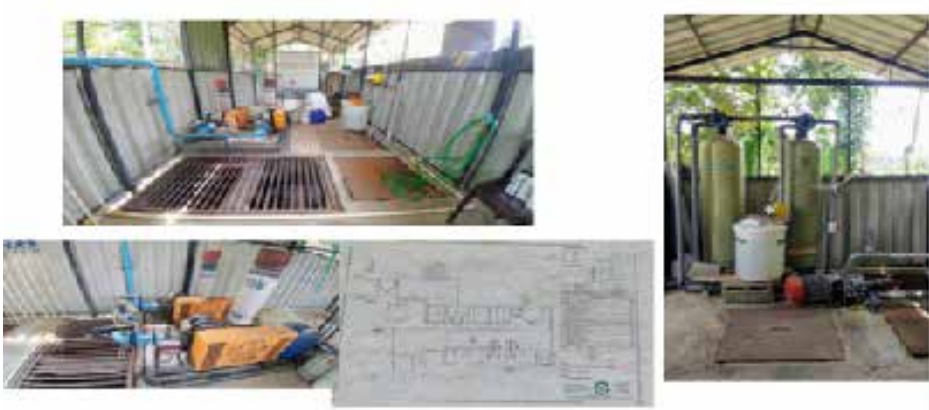
Figure 8: Wastewater Treatment Plant and Rainwater Harvesting
