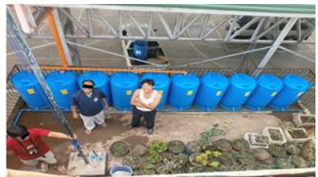
Figure 12: Rainwater harvesting using drums directly attached to roof downspouts
